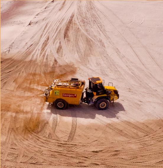
Hydratrac (dust suppression agent) being applied across the site to mitigate dust
